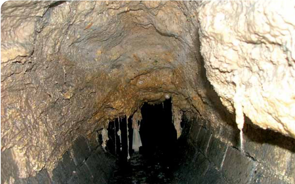
Fat beginning to block a sewer
